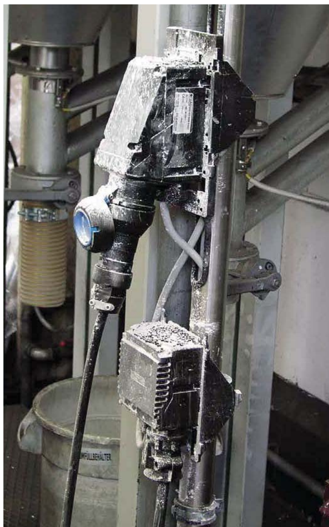
Example of dust Ex zone 21: Explosion-protected plug and socket and terminal box in the field
